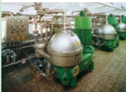
Process line with nozzle separators for the recovery of yeast.
