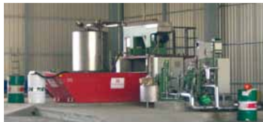
Waste oil treatment plant, Spain
