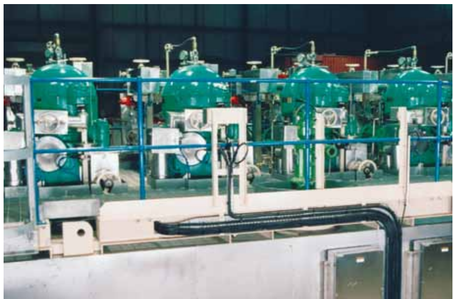
Cat fines removal plant in special design
