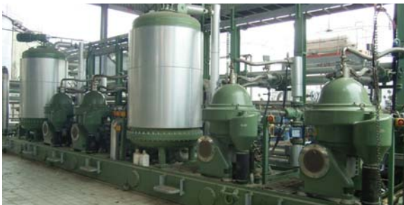
Module for heavy fuel oil washing
