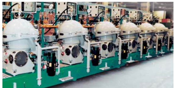
Module with six separators for naphtha
