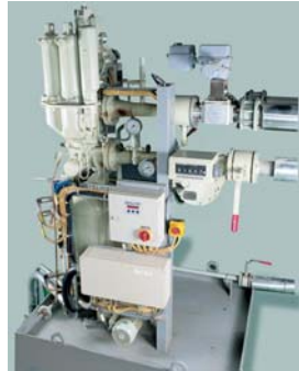
Fuel oil management module
