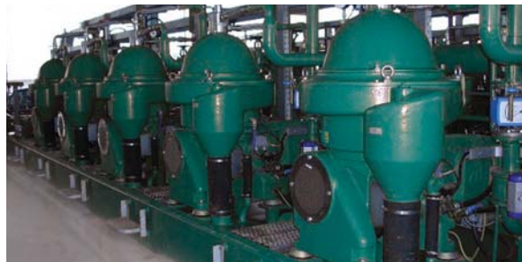
Module with six separators for distillate
