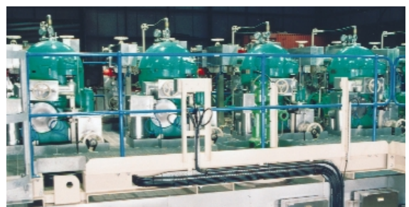
Centrifuge plant for cat fines separation
